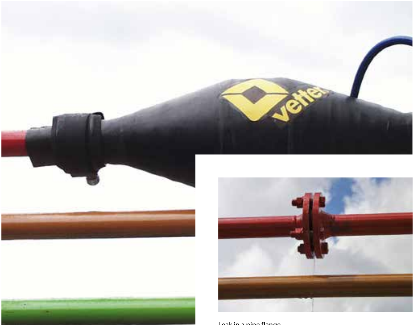
Leak in a pipe flange
